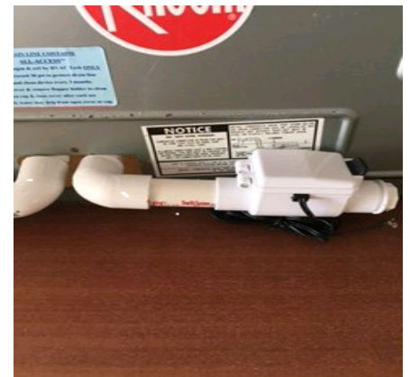
AA1-FS PLUGGED ON SECONDARY DRAIN PAN OUTLET
