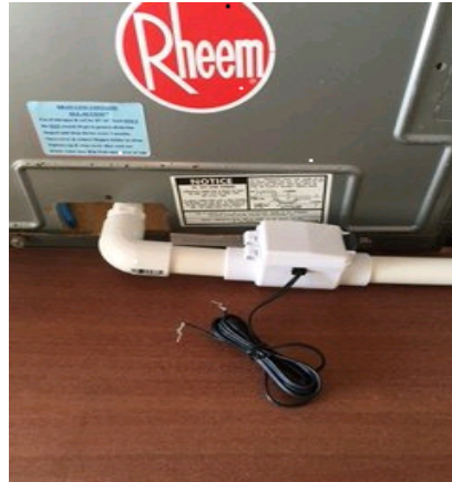
AA1-FS INSTALLED INLINE
